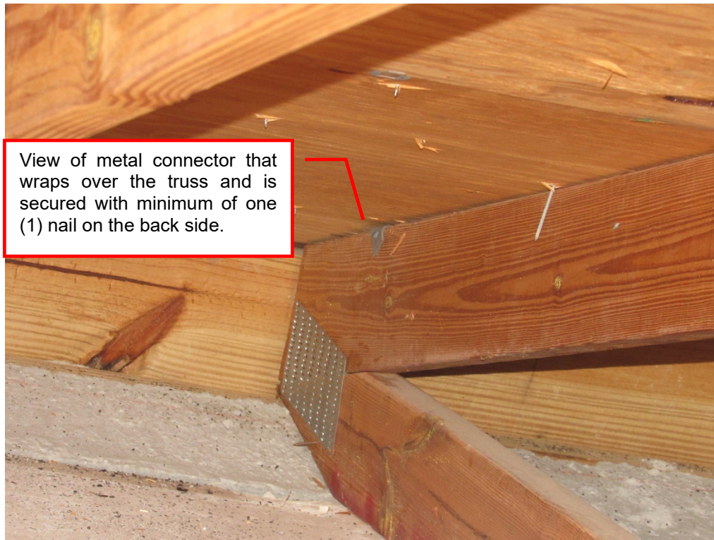
View of metal connector used on Roof to Wall attachment (per question 4).
