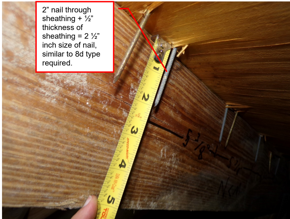
View of nail used on sheathing attachment (per question3).
